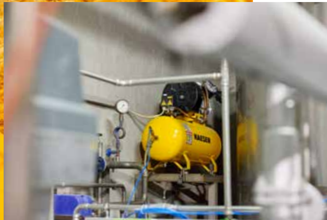
The Friedmann brewery has relied on compressed air from KAESER reciprocating compressors for many years.
