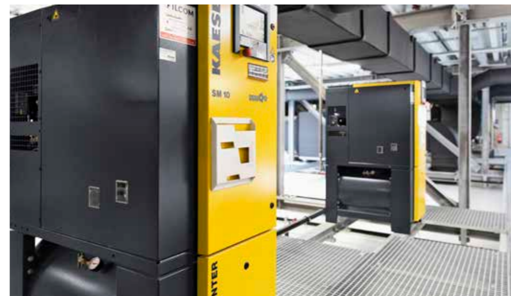
Two AIRCENTERS are installed at the new logistics centre.
