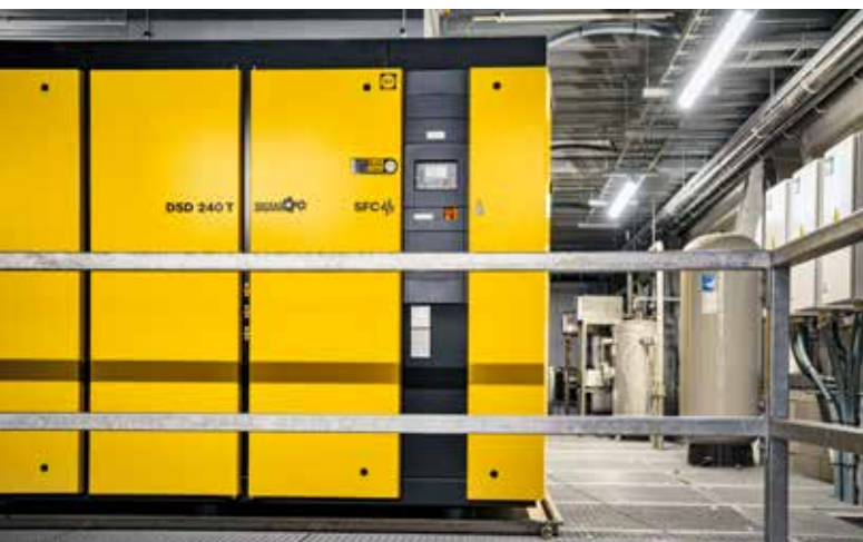
Three variable-speed DSD 240 T SFC rotary screw compressors with integrated dryers ensure a reliable supply of compressed air at the plant.
