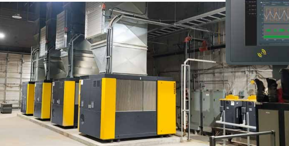
The frequency-controlled rotary screw compressor covers peak demand, while the three fixed-speed rotary screw compressors cover the base load.
