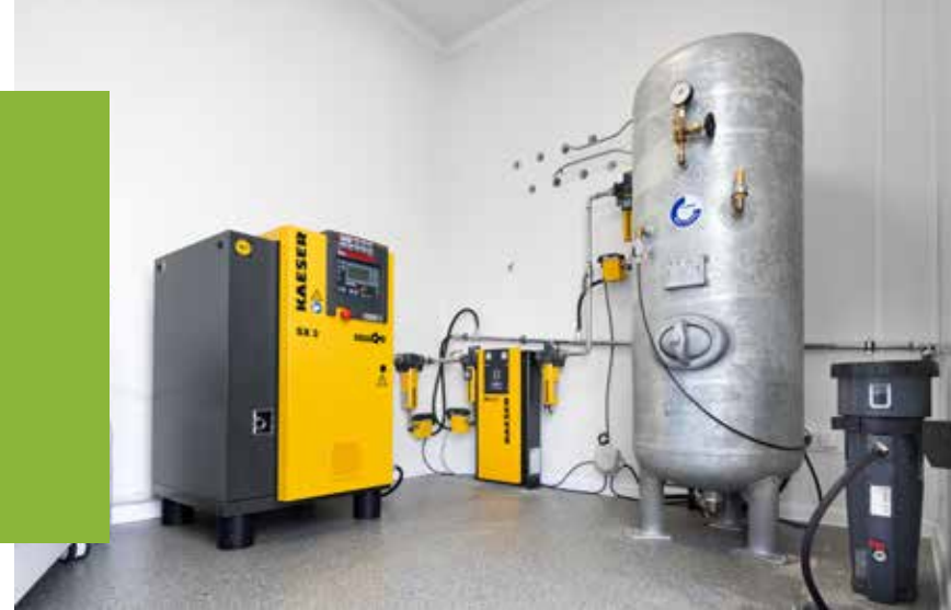
The SX 3 rotary screw compressor is accompanied by sophisticated compressed air treatment and a 250-litre air receiver.
