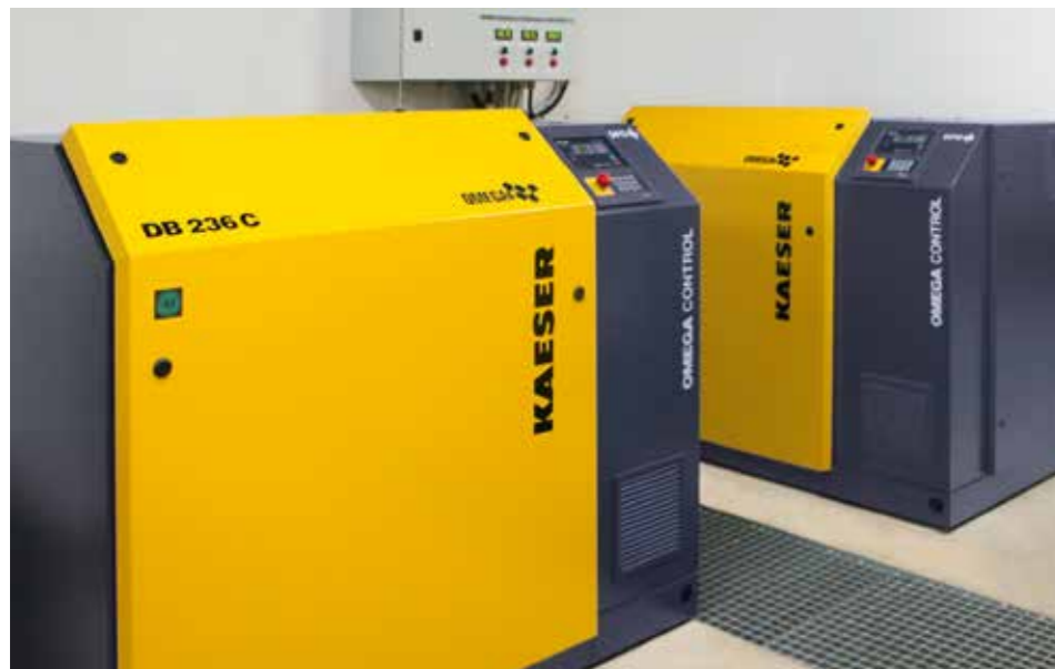
One of the key pillars of successful fish farming: a reliable oxygen supply from KAESER rotary blowers.
