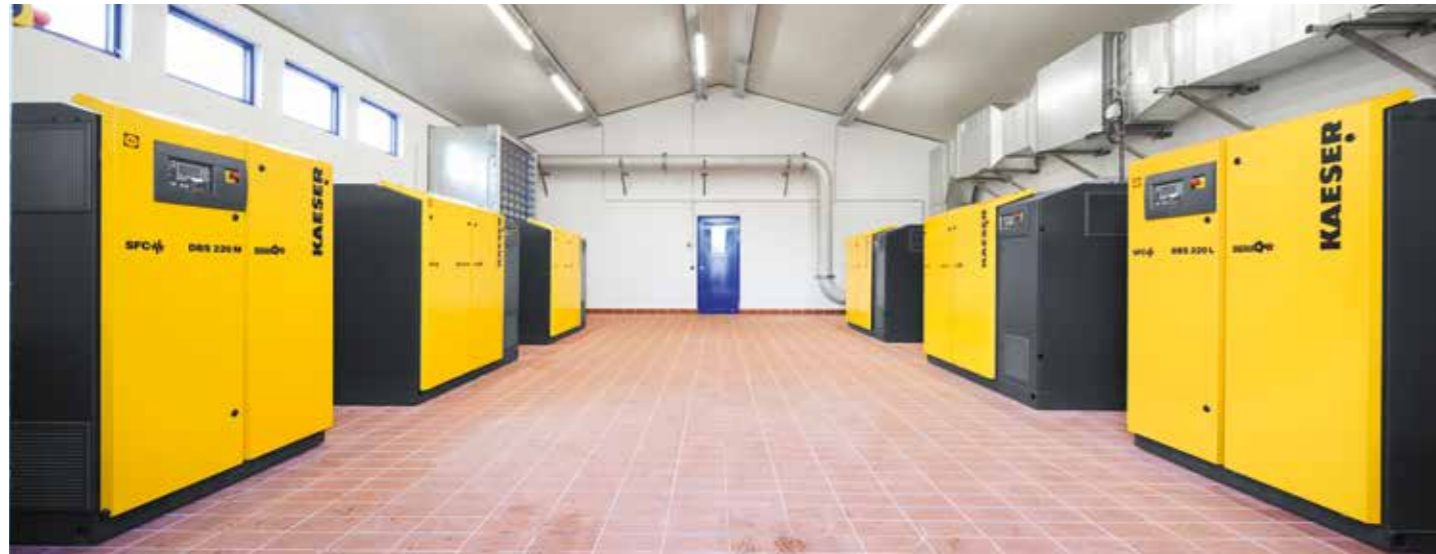
The blower station at the Lachen-Speyerdorf wastewater treatment plant, with its high-efficiency rotary screw blowers from KAESER KOMPRESSOREN.
