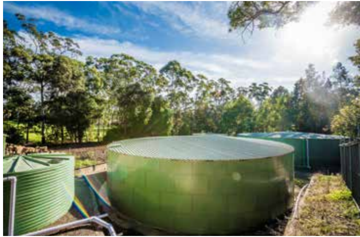
The water recycling plant supplies the club with its own source of irrigation water.
