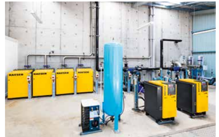
Four COMPACT-series rotary lobe blowers from KAESER are used to deliver process air for the membrane bioreactor.
