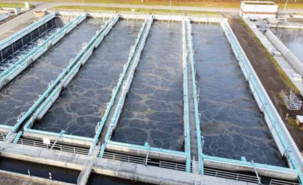
Compressed air is used to supply oxygen for the microorganisms active in the clarification tanks.
