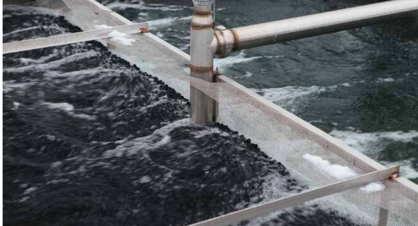
Nitrification ponds also need a lot of air from rotary blowers.
